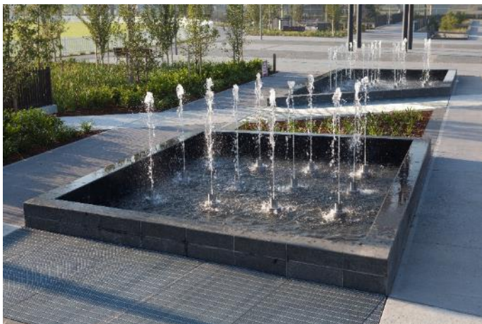
Thornton Development - Penrith NSW 2750 Landcom (Automatic Irrigation System & Public Domain Water Feature)
